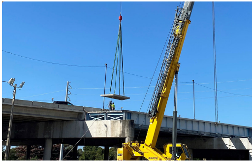
Bridge deck removal on I-395 to allow for new bridge foundation construction.
