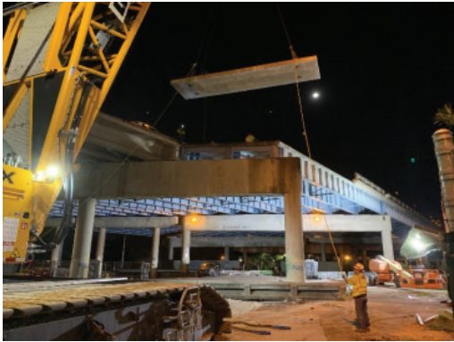
Removal of I-395 roadway deck over the FEC railroad track to allow new bridge foundation construction.
