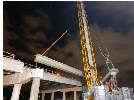
Erection of bridge beam for SR 836 widening over the eastbound SR 836 ramp to NW 17 Avenue.
