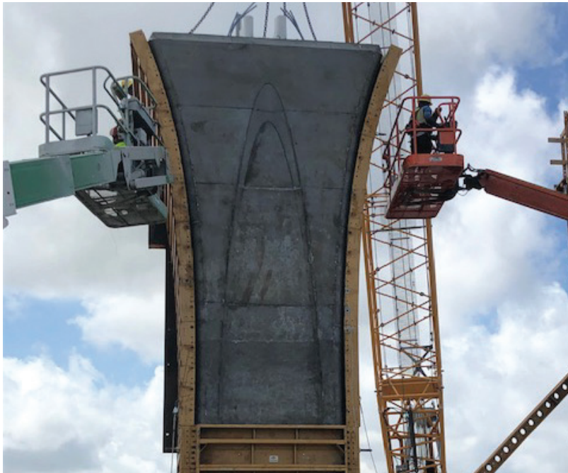
Crews removing the forms from a completed support column for the future I-395 westbound connector road.
