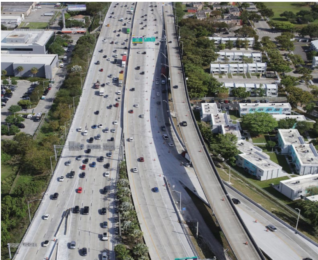
New concrete pavement on the SR 836 and I-395 ramp lanes to northbound I-95
