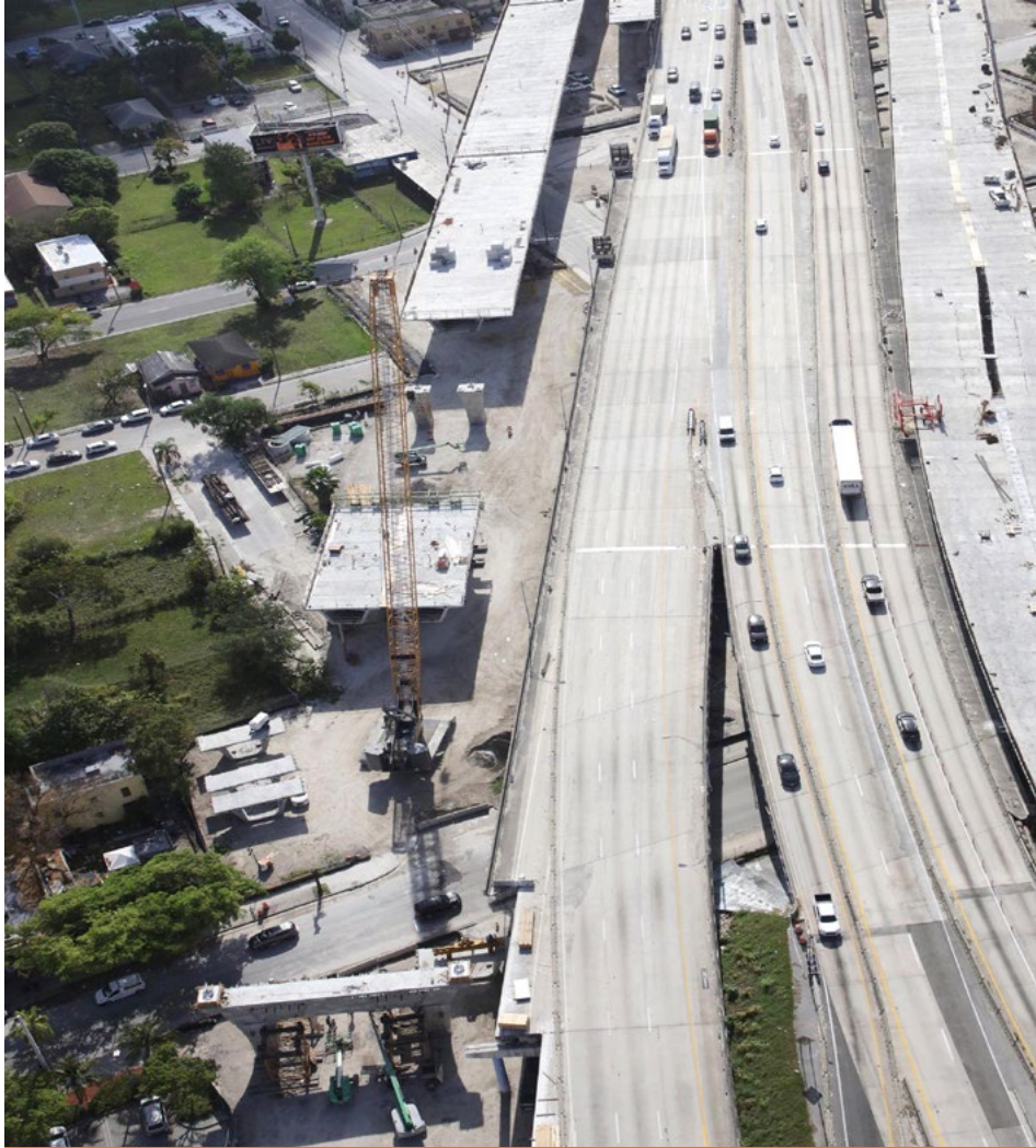
Installation of segments for a new section of westbound I-395 between NW 1 Place and NW 3 Avenue
