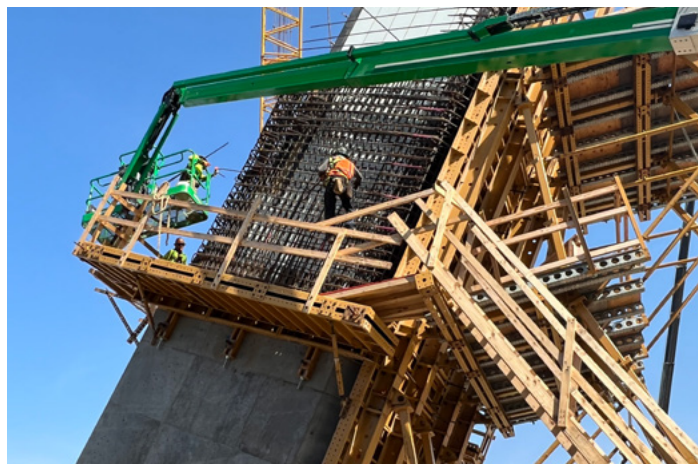
Ongoing preparations at one of the arches under construction for the second cast in place starter arch
