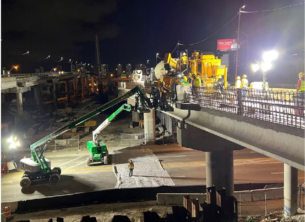
Crews slip forming the traffic railing for the widening of the eastbound SR 836 ramp to northbound I-95
