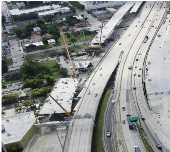
Ongoing installation of bridge segments adjacent to NW 3 Avenue for the new I-395 westbound local access roadway
