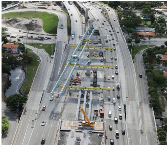
Fully assembled bridge cap and beam lifter just west of NW 17 Avenue at SR 836
