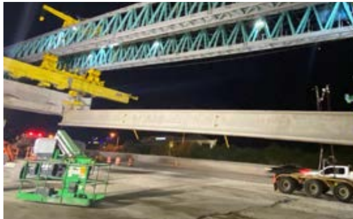
SR 836 beam and cap segment lifter installing a beam. To view an animation of how the bridge beam and cap segment lifter works, CLICK HERE .
