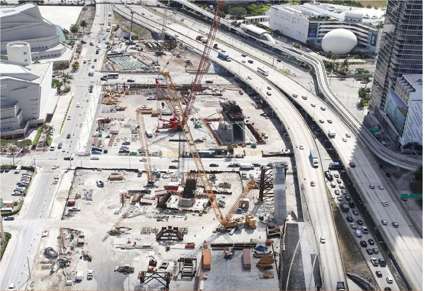
Signature bridge footprint showing four arches and the center pier support currently under construction
