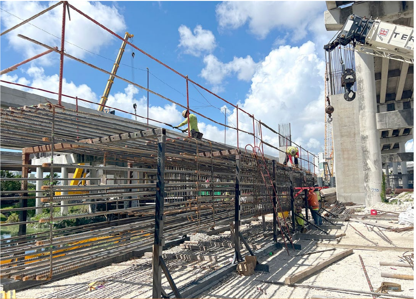
Crews tying reinforcing steel for a new bridge pier for the SR 836 double decked roadway
