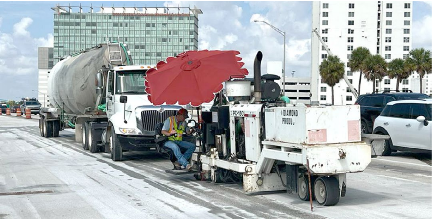
Diamond grinding of new concrete pavement on eastbound SR 836 at NW 12 Avenue
