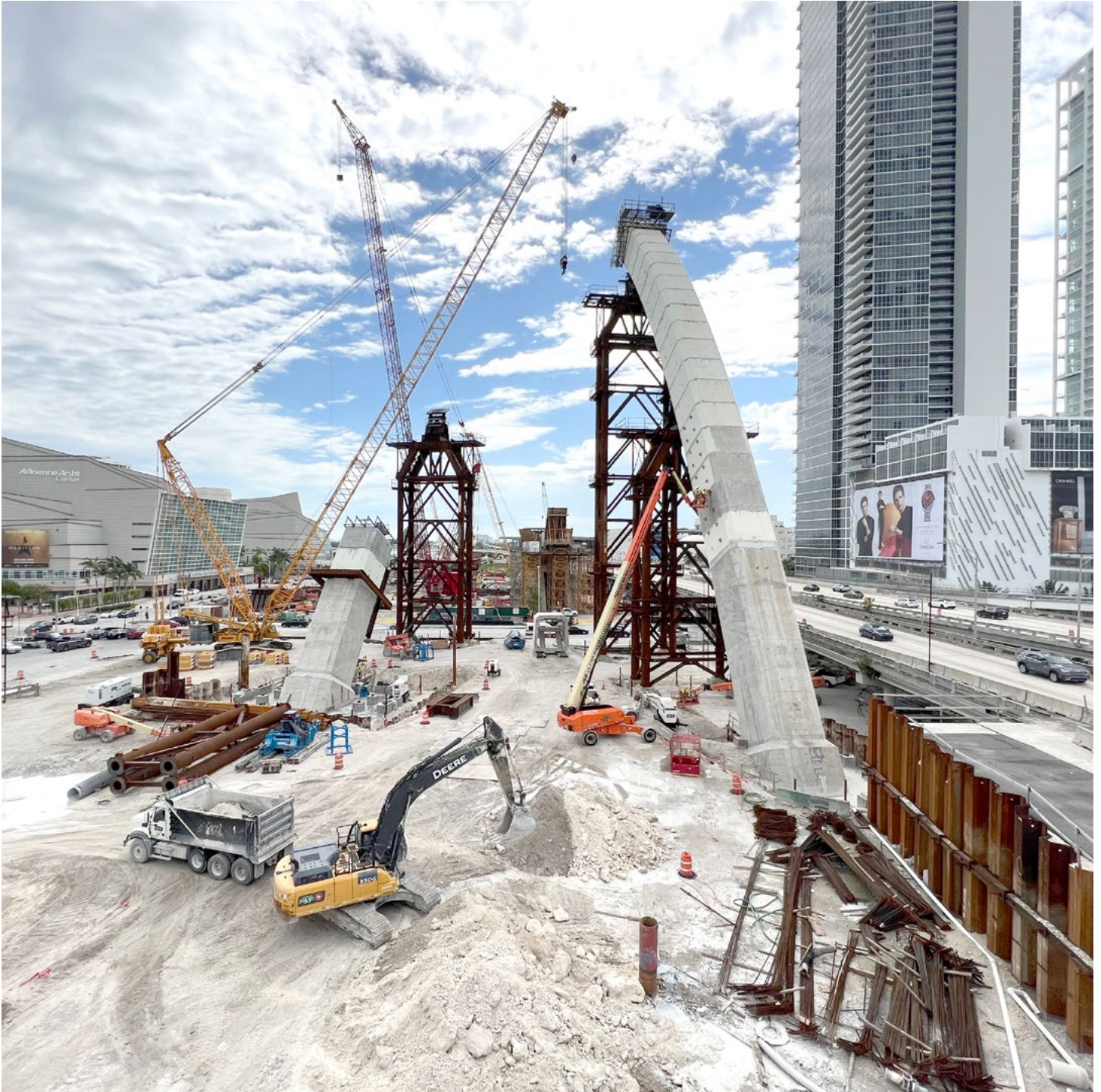
Ongoing signature bridge construction from west of NE 2 Avenue to east of Biscayne Boulevard
