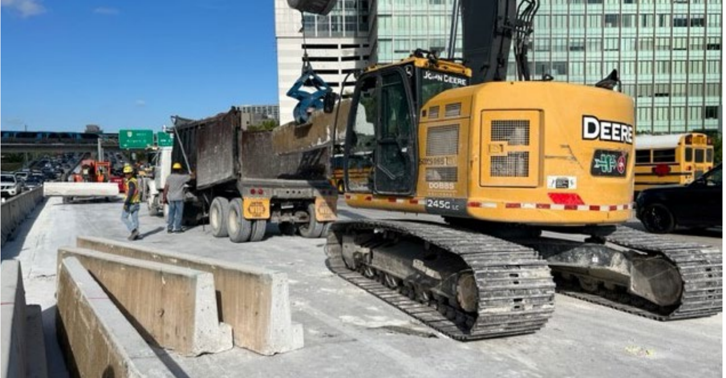
Ongoing demolition of the median on SR 836 from NW 12 Avenue to I-95 for construction of bridge foundations
