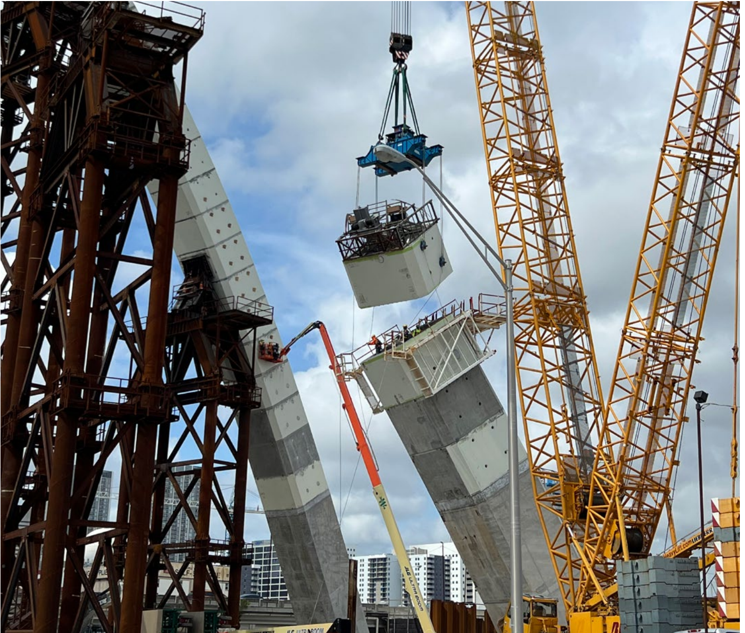
Installation of a precast arch segment for the I-395 signature bridge just west of NE 2 Avenue
